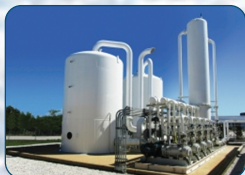
Liquefaction, Condensation, Storage Handling and Vapour Recovery
